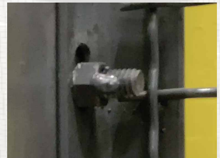
Tamper-proof hardware on inside of cage.
